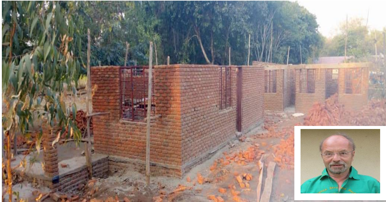
Chilumba village clinic taking shape. Insert, Dr Holger Keppel. Who has been instrumental in raising funds for projects being implemented by URAC in Chilumba, Karonga. Pic. Solomon Salanga, URAC
