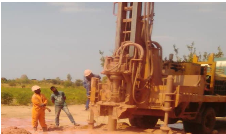
Drillers working on the borehole at Bobu Village, Ngala, Nkhota-kota. Pic. Wongani Chunga, URAC
